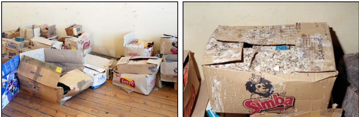
Figure 2.9 Bird droppings on photographic material storage boxes.
